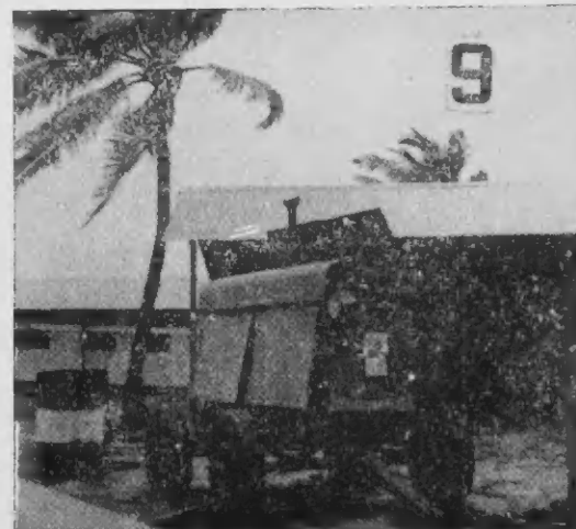
The problem of how to supply power was ingeniously solved when CB&I set up a welding generator. Residents must be careful, not to use too much electricity at one time.
